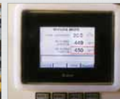
6 Control panel display
